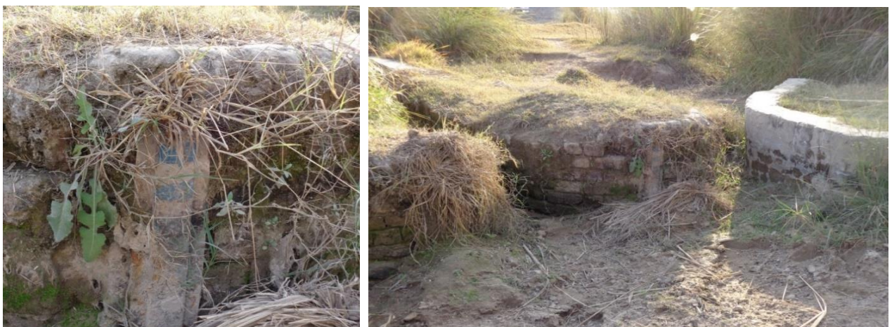
Figure 10. Poor tail maintenance
