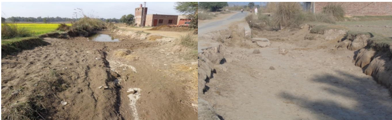
Figure 5. Poor condition of Joyanwala distributary prism
