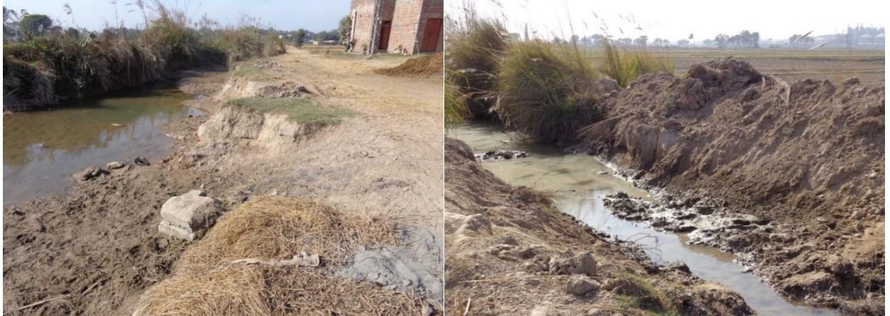
Figure 3. Inadequate bank maintenance on Joyanwala distributary
