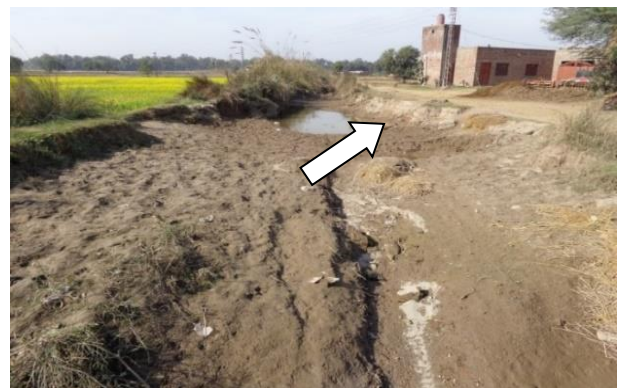
Figure 9. Encroachment on Joyanwala distributary.
