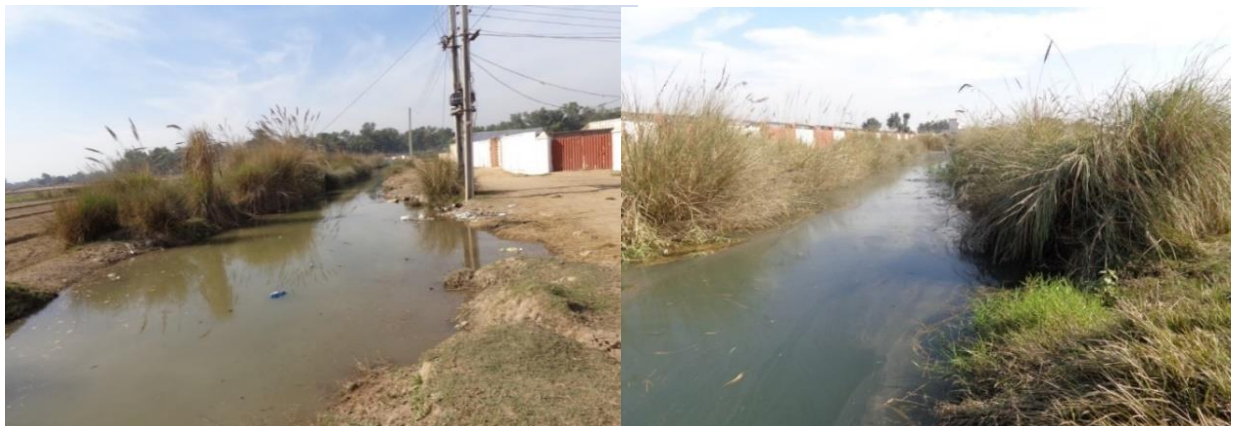
Figure 4. Inadequate free board on Joyanwala distributary
